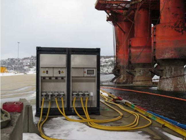
Fig. 3 – Photograph showing the shore power connection for offshore rig
