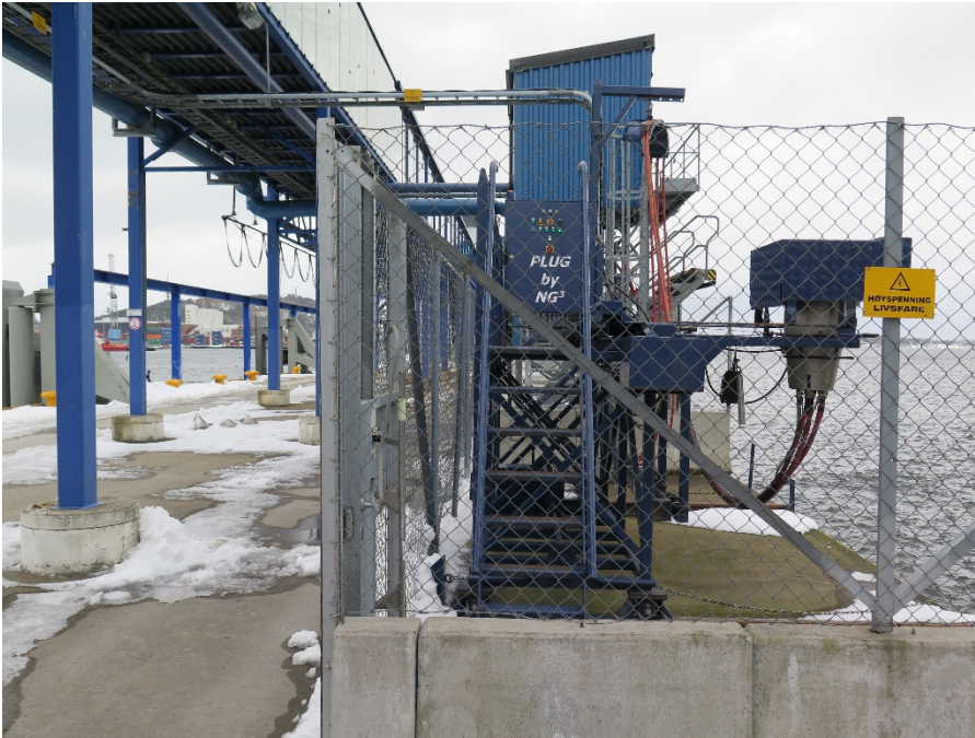
Fig. 2 – Photograph showing the shore power connection for passenger ship
